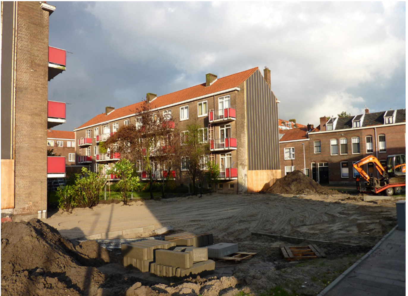
The Oude Tuinen after the demolition of the housing at the end of the block. A garden was planted and a greenhouse/shed called De Kas was built here. Stichting NAC.
