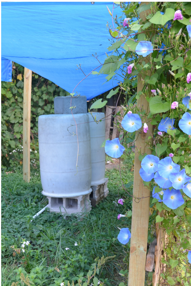
The rainwater harvesting system for the garden.
